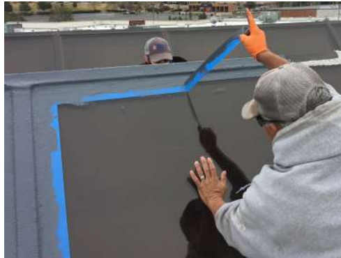
While the Sikalastic® RoofPro resin is wet lay in precut lengths of Sika reinforcing scrim and embed with a wet roller or brush to ensure full saturation and conformation to the substrate.
