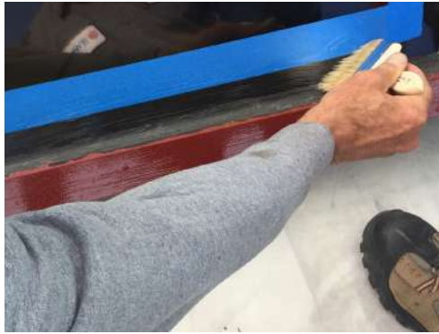
Prime frame and mullion with Sikalastic® EP Primer. Then, mask off skylight 2 inches from the mullion and prime glass with Sikalastic® Clearglaze.
