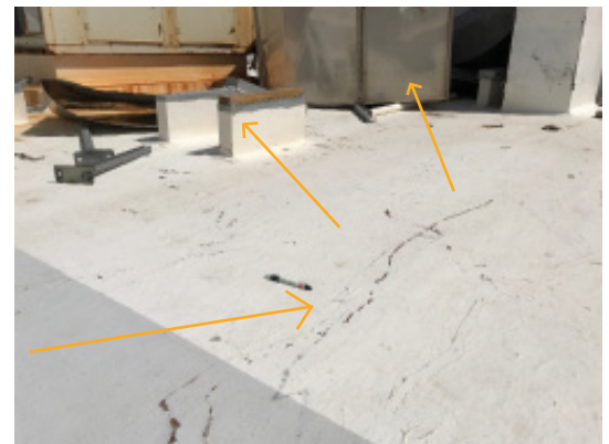
Skid Marks in RoofPro membrane from airborne debris during hurricane
