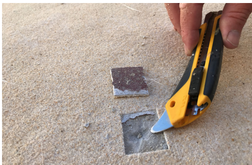
A closer look at gouge marks in RoofPro membrane
