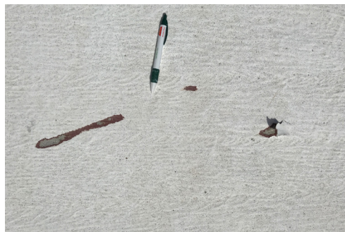
Still bonded after 185 mph winds from Hurricane Irma - only gouges in top of membrane
