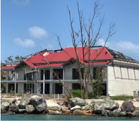
Coastal home with torn off roof
