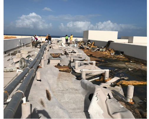
Torn off loose laid membrane system
