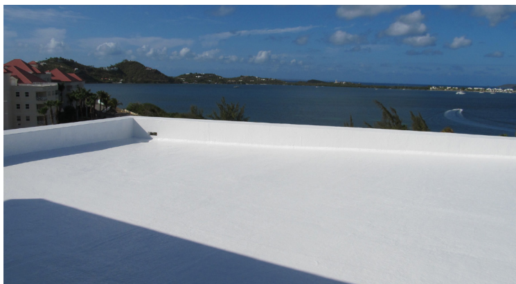
Sikalastic® RoofPro membrane on the medical building roof at the American University of the Caribbean in St. Martin
