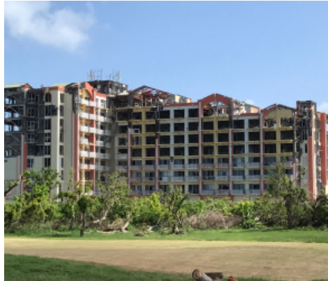
Hurricane damaged building
