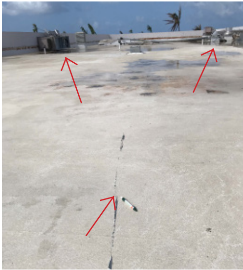
Mechanical equipment that became airborne on the CEP building during the hurricane caused skid marks in the RoofPro membrane
